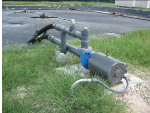
Plate 8. Bank mounted AIA Taeration system. System has air vents and water intake/out-take vents.
