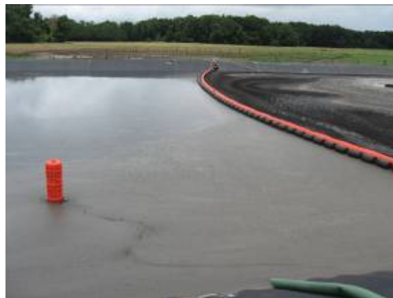
Plate 9. The lagoon filled and overflow structure in operation
